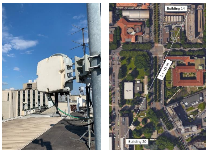
Fig. 1. The E-band Huawei link transceiver (left side) and the corresponding link path between Buildings 14 and 20 of Politecnico di Milano (right side).
